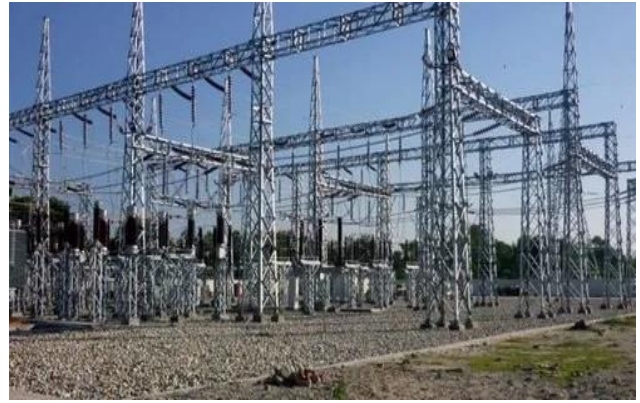
Power Utility's 132 kV Electrical Substation India
