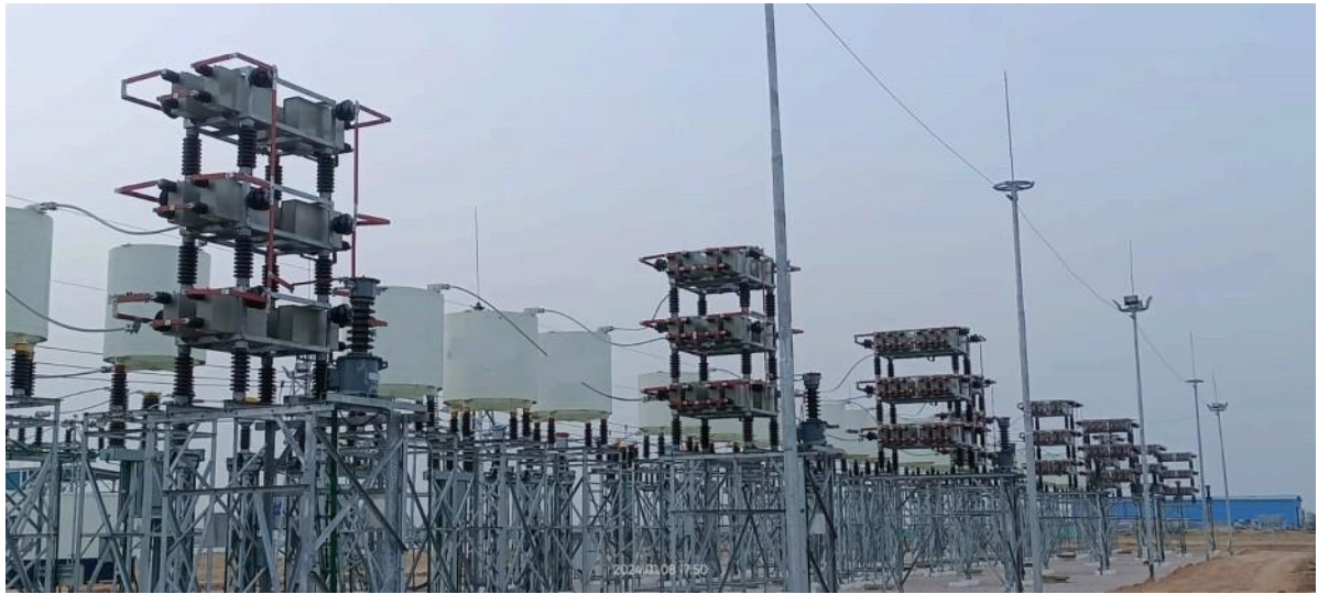
CosPower's Capacitor Banks at a Solar Power Plant at Bikaner, Rajasthan
