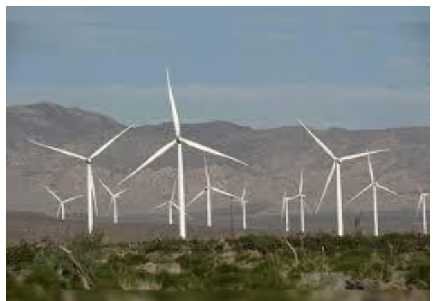
Wind Farm Power Plant
