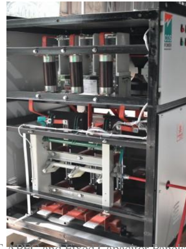
HT APFC and Fixed Capacitor Panels
