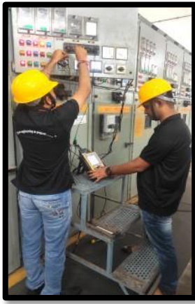
Harmonic and power studies at site by CosPower's Team drawing CosPower a company that offer complete solution in Power Quality Improvement
